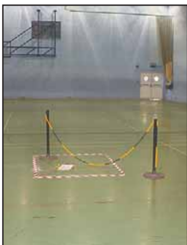
The damaged area of floor located close to the centre of the sports hall
