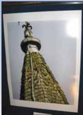
The spire before the repair works. Visit the church to see how it looks now!
