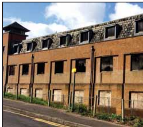
The dilapidated building currently on the site, Garrod House.
