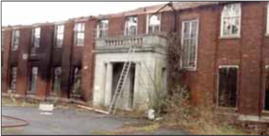
The charred facade of the Officers' Mess after the fire.
