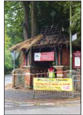
The St. Luke's lych gate after the fire.
